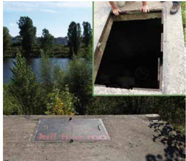
Fig. 9. The cover of a sewer manhole that guides wastewater to the sewage plant, and the open sewer, a 6 m deep trap for snakes. Photo: MIKULÁŠ VELENSKÝ and KONRAD MEBERT
