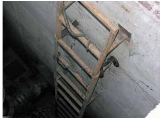
Fig. 10. A ladder leading down the sewer manhole with adult dice snakes sitting on it. Photo: MIKULÁŠ VELENSKÝ
